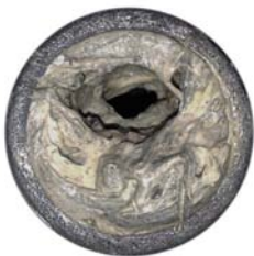
FIGURE 1 - Debris inside suction line builds over time.
