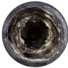
FIGURE 2 - Debris inside suction pipe after Bio-Pure Microbial Cleaning.
